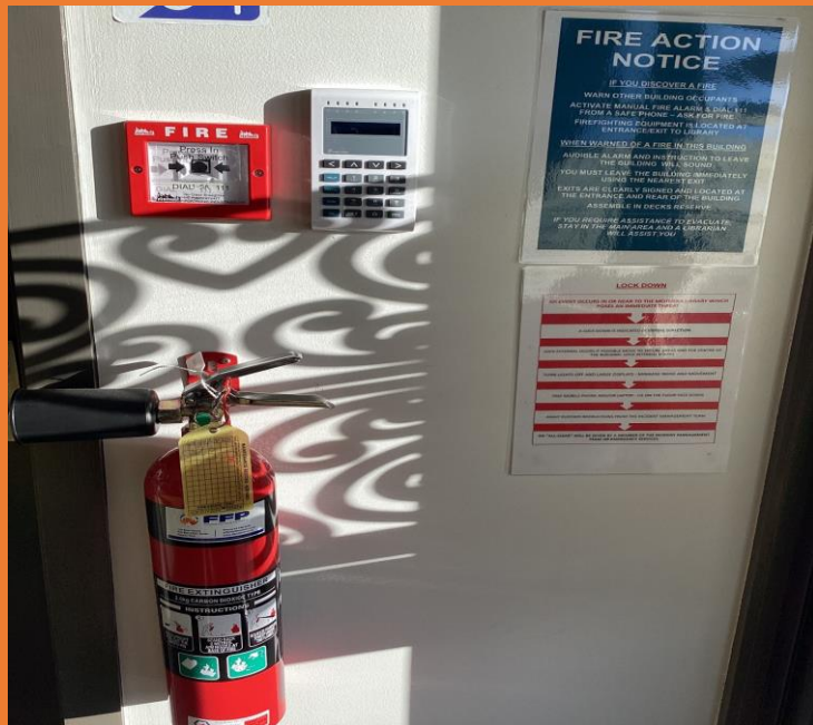
The fire alarm, fire action notice and fire extinguisher are located just inside the afterhours door.
