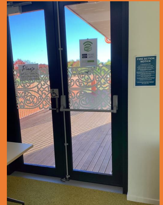
Fire exit Decks Reserve
