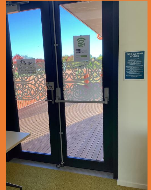
Fire exit Decks Reserve
