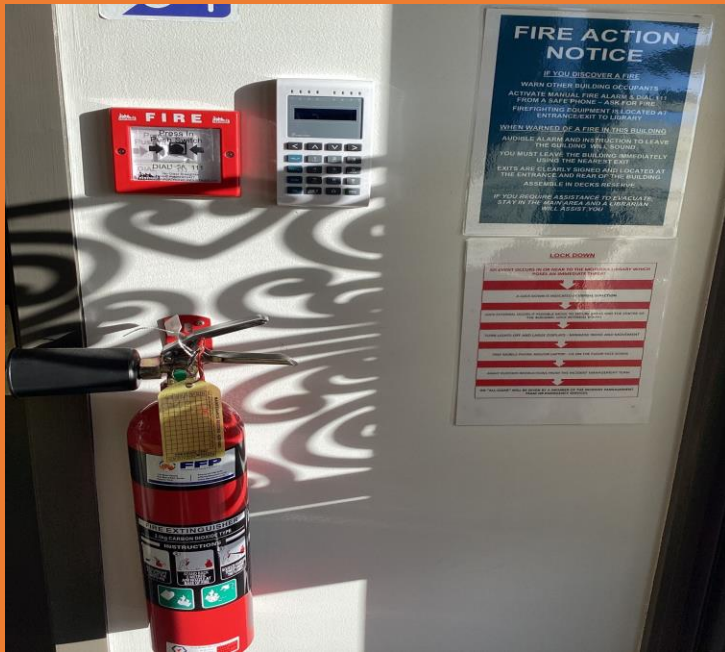
The fire alarm, fire action notice and fire extinguisher are located just inside the afterhours door.
